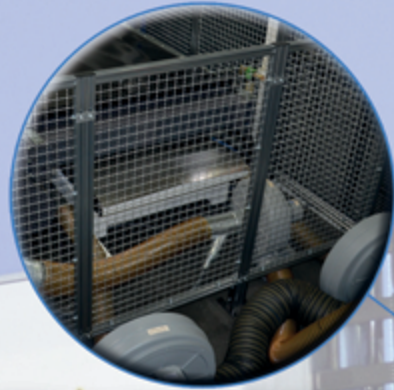
3 Exhaust ventilators to extract the cutting smoke
